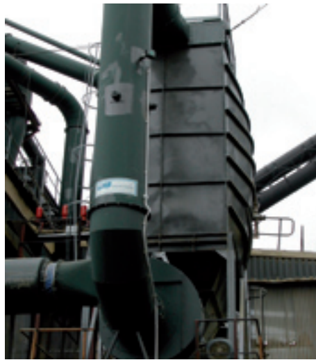
Filter down-time reduced by predictive maintenance
