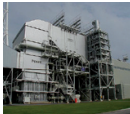
Flue Gas Desulphurisation Plant
