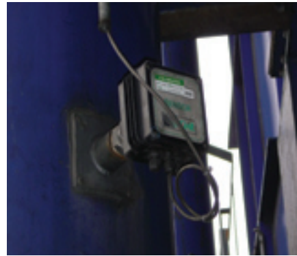
The interspace between Primary and Secondary HEPPA Filters monitored by an approved (MCERTS, TUV) Electrodynamic Sensor
