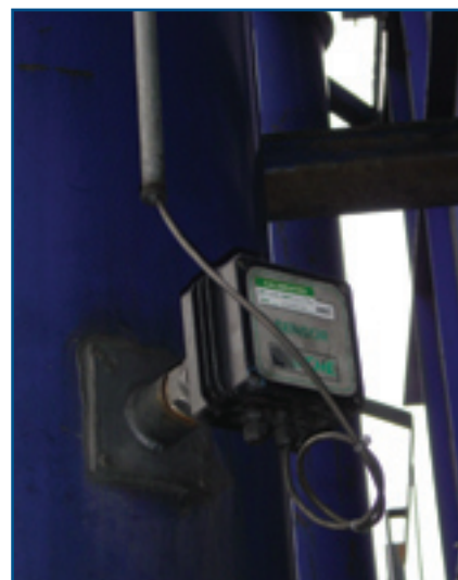
Electrodynamic Sensor installed in bag house outlet
