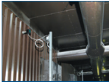
Electrodynamic sensor installed directly in Baghouse compartment wall
